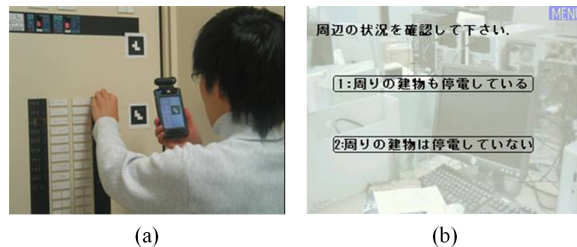
Figure 12: The user checks the switchboard using a PDA. Figure (b) shows an example of a dialogue (in Japanese Kanji). It directs the user to look around at his/her surroundings.
